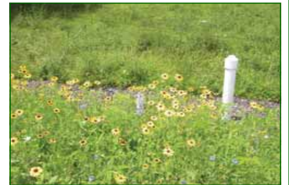
Top to bottom: Infiltration trench to decrease nonpoint source pollution and reduce downstream velocity and flooding during installation, two weeks after, and two months after.
