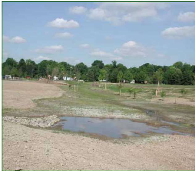
Above: Detention/recharge area in the initial stages of creating the wetland stormwater system.
