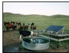
Solar powered remote watering system
